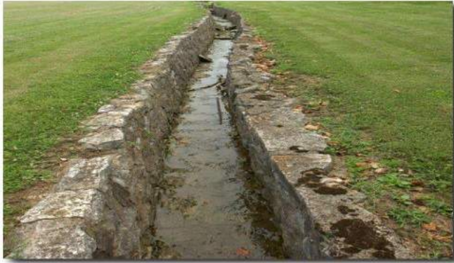
Figure 4. An open surface drain used to evacuate excess surface water
