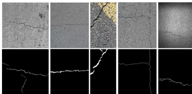
Fig 1 : Road crack with segmented results
