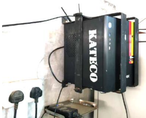
Figure 1: iBox installed in a senior high school (Cullen, Mallett, & Murphy, 2019).
