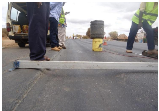
Figure 1.2: Rutting on Mombasa Road, Salama Town
