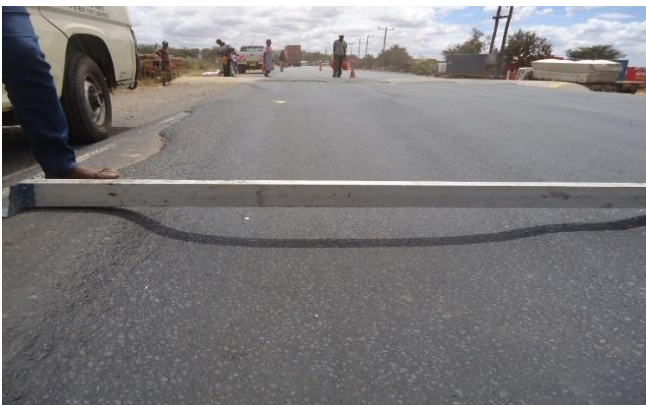
Figure 1.4: Rutting on Mombasa Road, Emali Town
