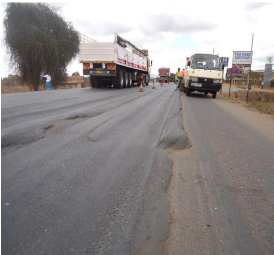
Figure 1.5: Rutting on Mombasa Road, Makindu Town
