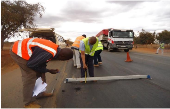
Figure 1.3: Rutting on Mombasa Road, Sultan Hamud Town
