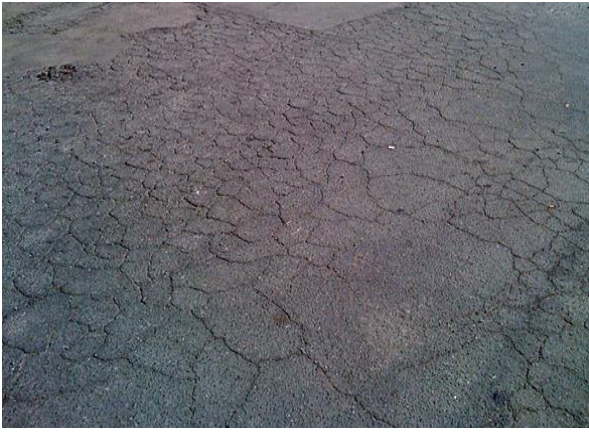
Figures 1.6 (b): Pavement cracking of asphalt pavement
