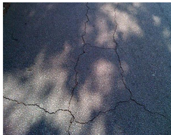
Figures 1.6 (a): Pavement cracking of asphalt pavement
