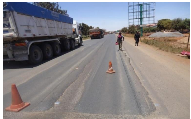
Figure 1.1: Rutting on Mombasa Road, Machakos Turn off
