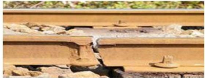
Fig. 1: Crack on track
