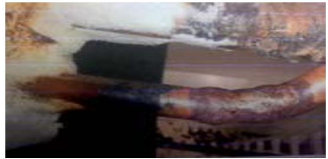
Figure 6 : Improper installed pipe due to poor workmanship
