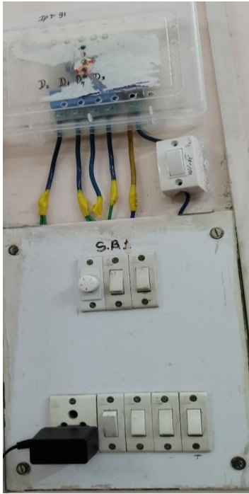
Fig: module connected with switchboard
