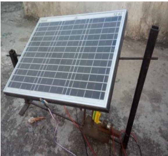
Figure 5 : solar panel tracking implementation
