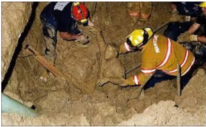
Figure 6 Deep Excavation trench collapse – Confined Space Entry
