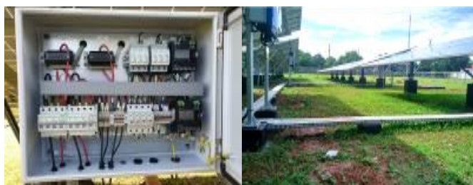
Figure 7. DC Distribution Side Condition of PV Power Plant I Source: PLN UPDL Makassar, 11/23/2021
