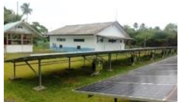
Figure 13. DC Distribution Side Condition of PV Power Plant II
