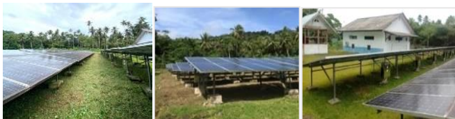
Figure 12. Solar Module Condition of PV Power Plant II
