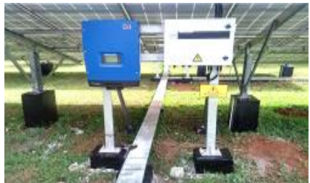
Figure 8. Inverter Condition of PV Power Plant I Source: PLN UPDL Makassar, 11/23/2021
