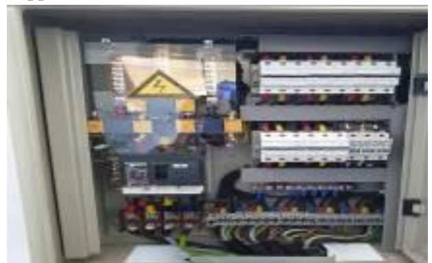
Figure 9. AC Distribution Side Condition of PV Power Plant I | Source: PLN UPDL Makassar, 11/23/2021
