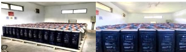
Figure 15. Battery Condition of PV Power Plant II Source: PLN UIW Maluku, 3/2/2022
