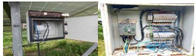
Figure 20. DC Distribution Side Condition of PV Power Plant III
