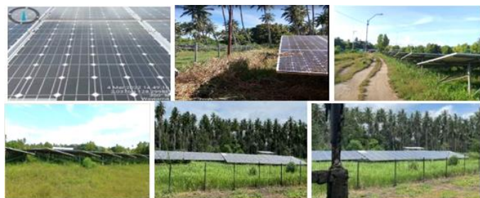
Figure 19. Solar Module Condition of PV Power Plant III
