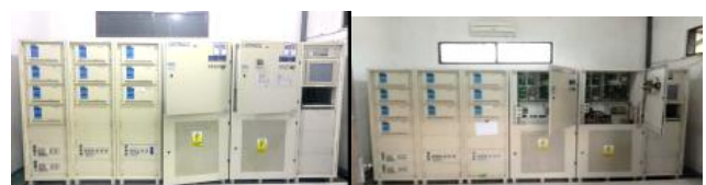
Figure 14. Inverter Condition of PV Power Plant II
