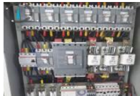
Figure 16. AC Distribution Side Condition of PV Power Plant II
