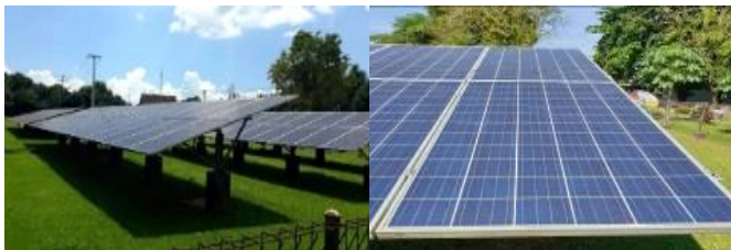
Figure 6. Solar Module Condition of PV Power Plant I Source: PLN UPDL Makassar, 11/23/2021
