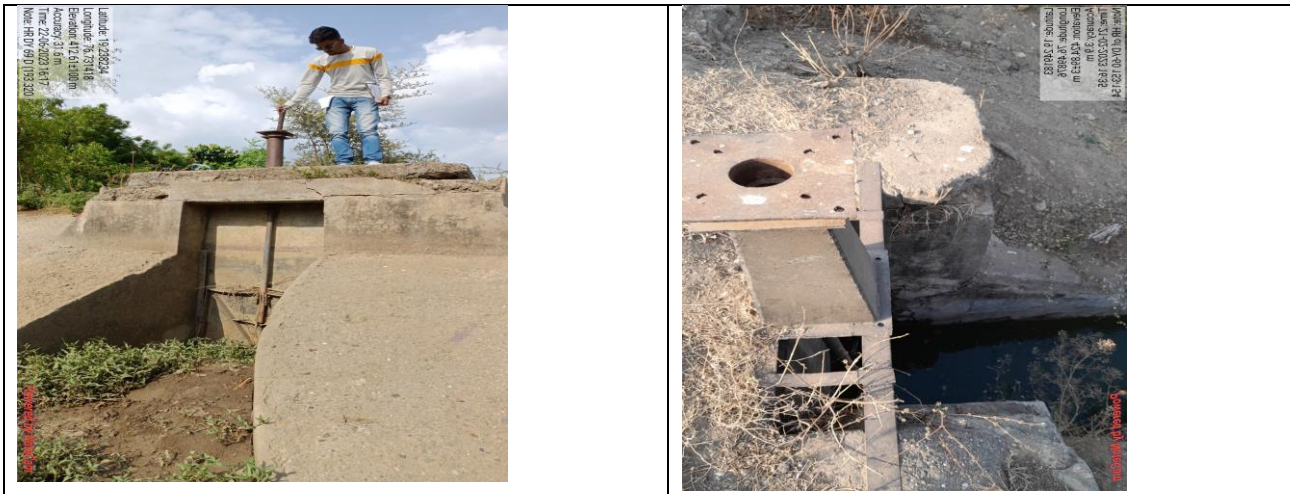
Figures showing the gate with vertical lift steel plate.
