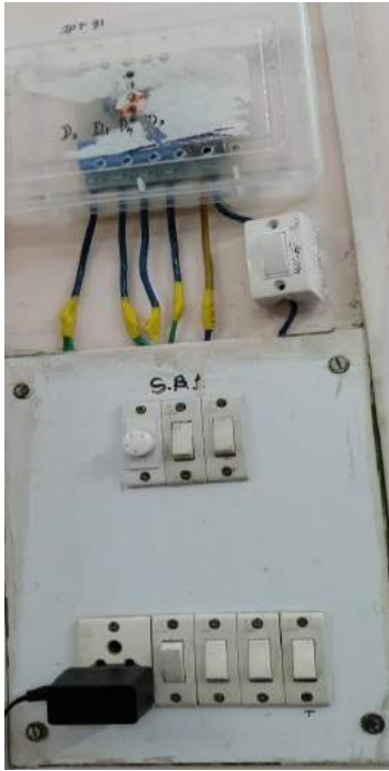
Fig: module connected with switchboard
