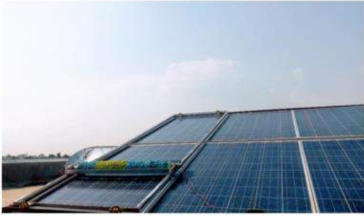
Figure 4 : solar panel cleaning using roller brush.
