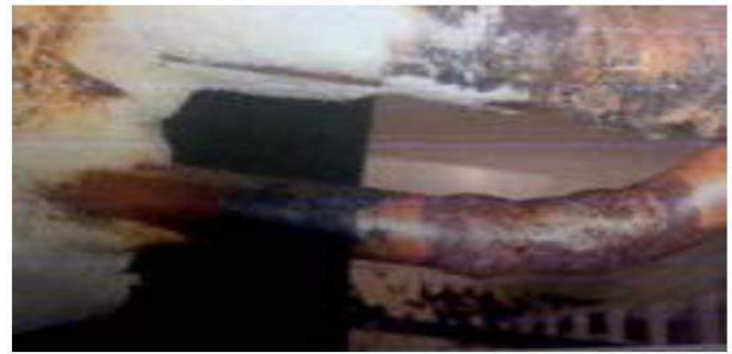
Figure 6 : Improper installed pipe due to poor workmanship
