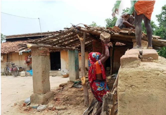
Fig 6 : Self made homes with wall thickness 30-40 cm
